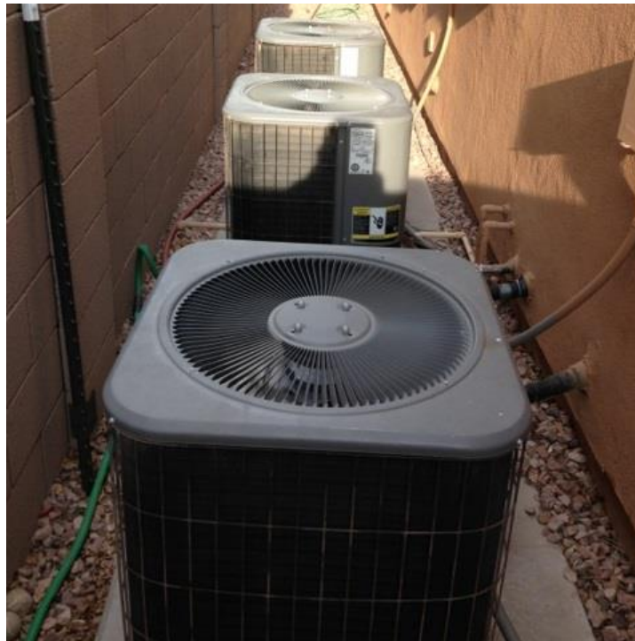
Fig. 1. Three 3-ton air conditioning units are required to cool my home in Phoenix where temperatures have been known to reach 120°F (or about 49°C) in the summer.
